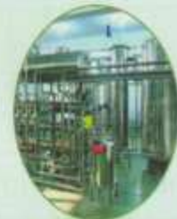
SHIVAY WATER PLANT
